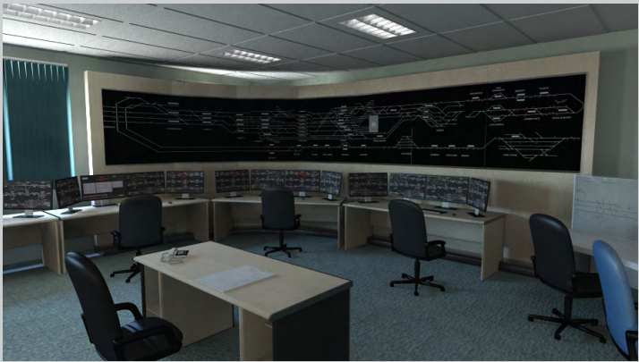
Operation Control Centre
